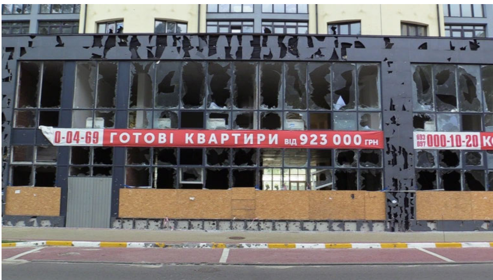
A sign saying ‘Complete apartments’ on a damaged building in Irpin, in
